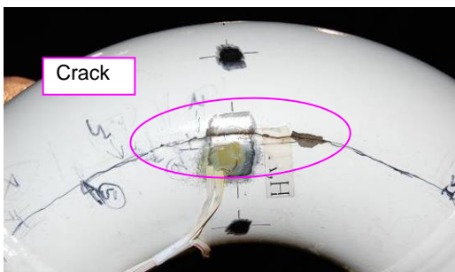
(b) The Axial Crack at the Flank of Elbow3
