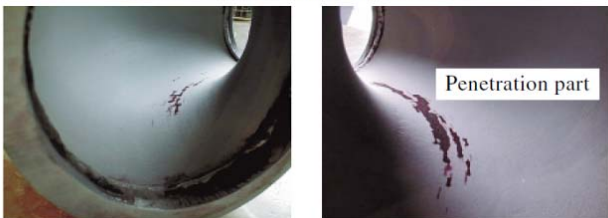
(b) Crack on side inner surface of Elbow2.
