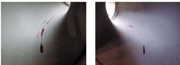
(a) Crack on side inner surface of Elbow1.
